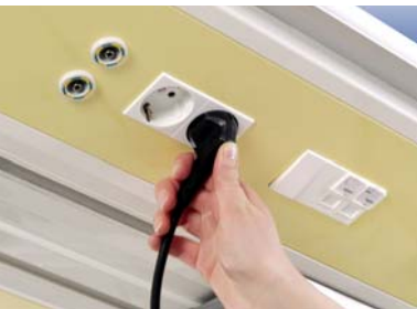
Electrical sockets and data interfaces; ergonomic connection angle
